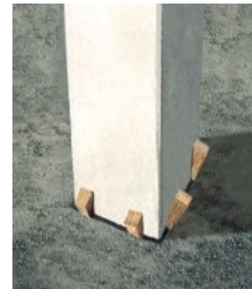
3. Place the column in the foundation and fill in the clearance of the filling material.
